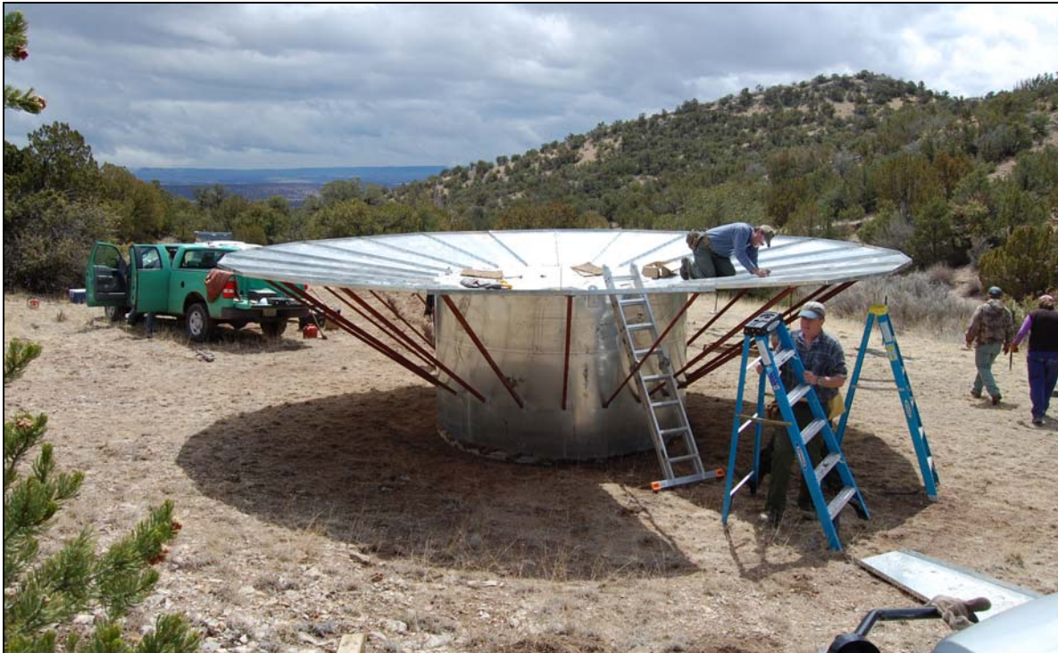
Volunteers for the Outdoors installed the Priest Trick Tank (CF-2009-009) in the southern Manzano Mountains, Cibola National Forest near Mountainair.
