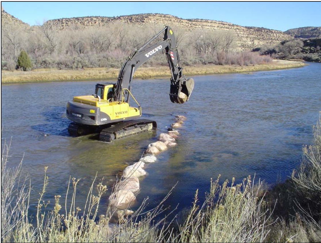
Farmington BLM Field Office personnel partnered with the HSP and many others to install boulders as resting places for trout on the San Juan River, near Navajo, NM. Photo courtesy of John Hanson, BLM.
