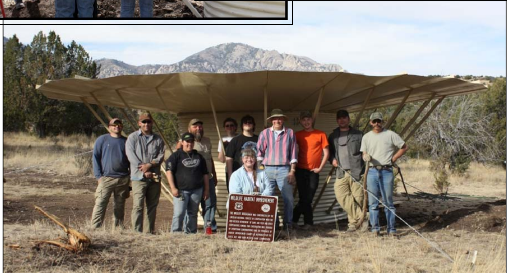
Sawset Trick Tank (SEF-2010-004). Cost of installation of trick tank was offset by local volunteers and members of Sierra Blanca Chapter of RMEF.
