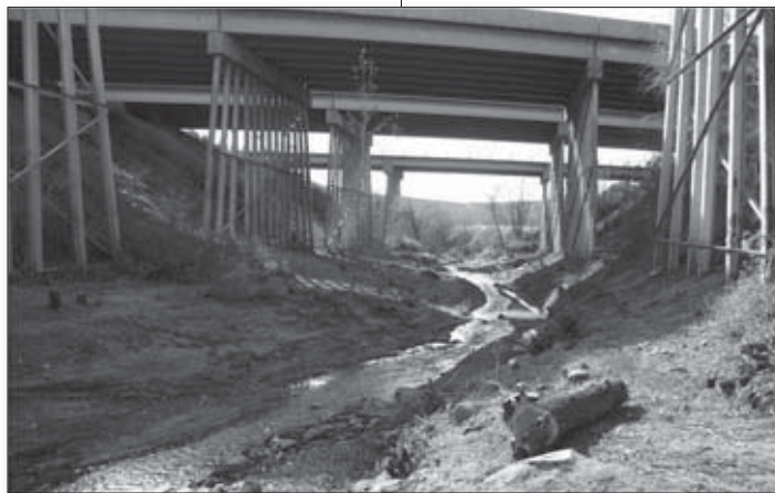
This underpass at Tijeras Canyon provides a corridor for wildlife moving across Interstate 40 east of Albuquerque. Photo courtesy of Tijeras Canyon Safe Passage Coalition.
